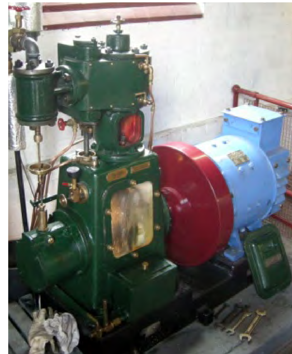
Reader steam engine driving GEC generator at Coleham Pumping Station (Courtesy gracesguide.co.uk).
